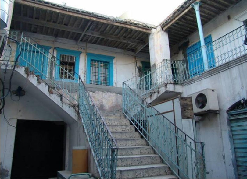
Figure 8: A house in Tripoli castle with the addition of inappropriate material and utilities
