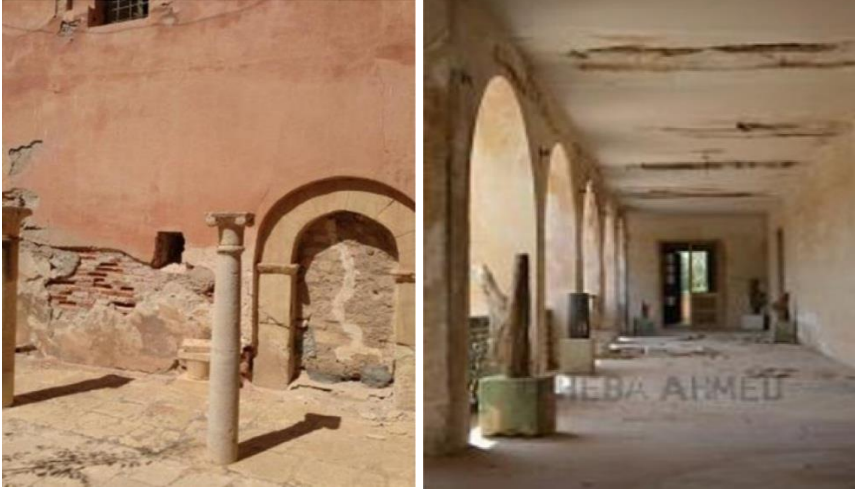
Figure 2: Deep cracks in the walls and slabs of Red Saraya
